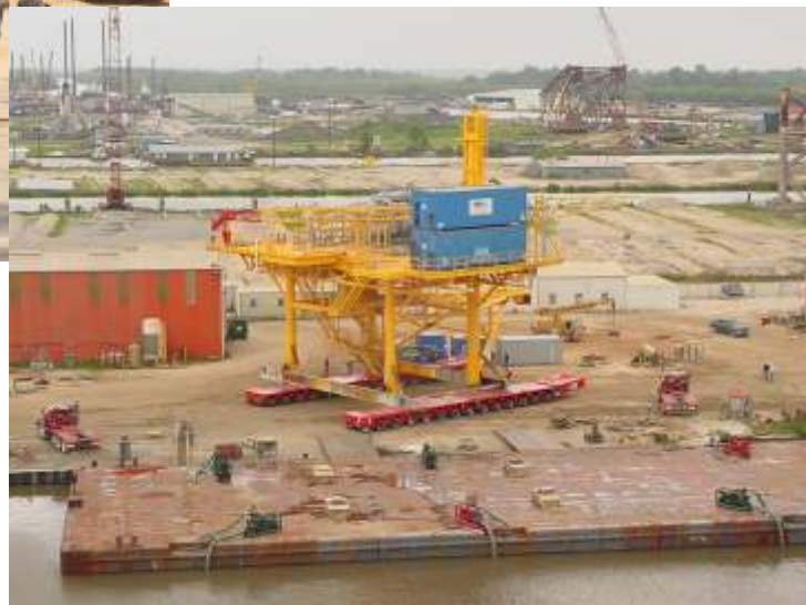
Pic. 61 PSP module transporter with drilling rig module before being loaded onto a barge
