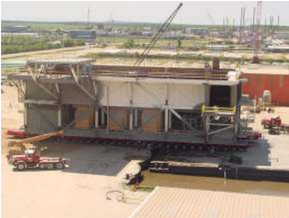
Pic. 58 PSP module transporter with drilling rig module before being loaded onto a barge
